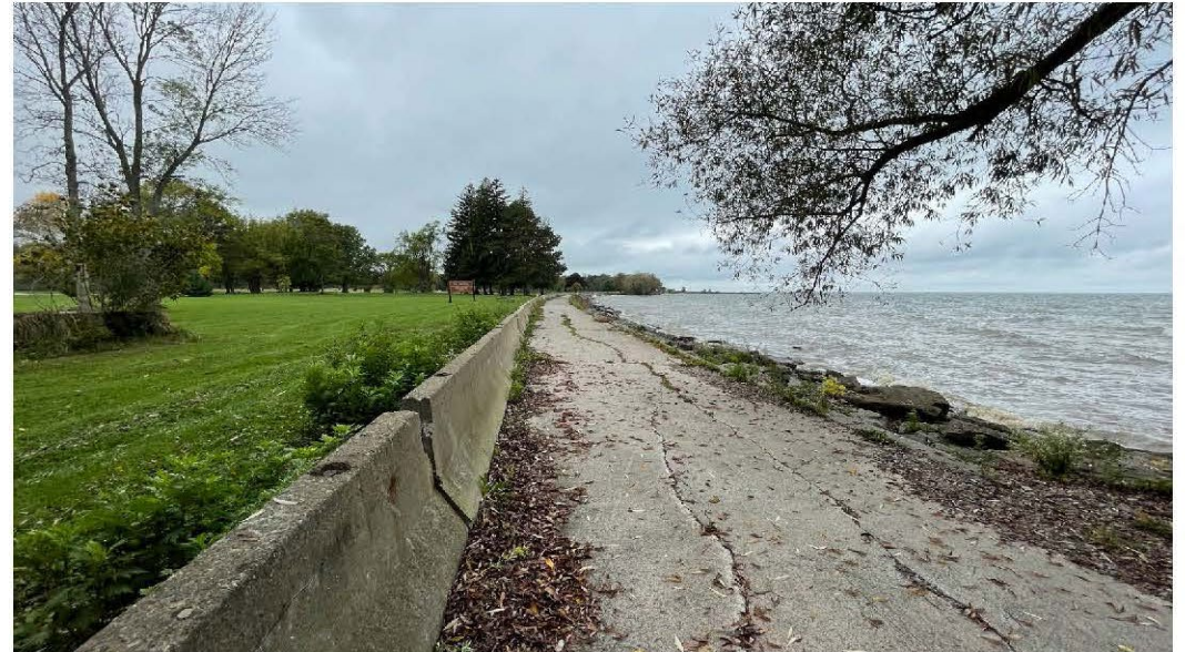
Prior flood / erosion control efforts (barrier wall), pavement undermining
