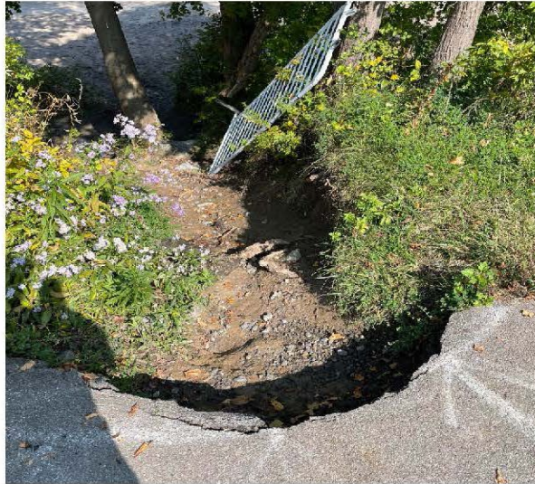
Trail pavement undermining
