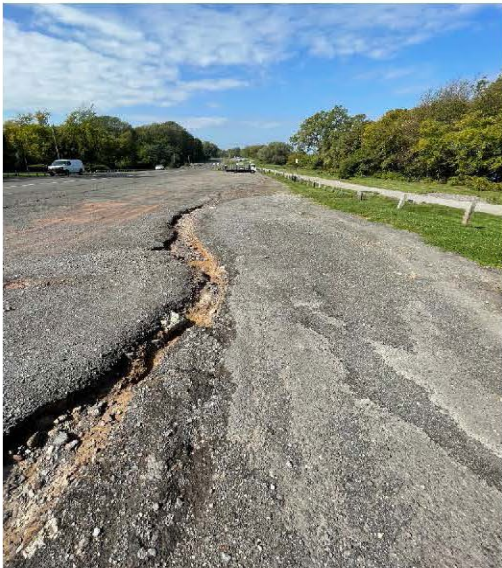
Parking lot erosion
